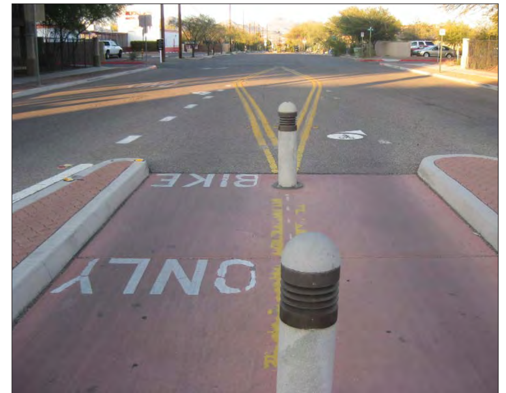
Wayfinding markings, striping, and signage at toucan crossing
